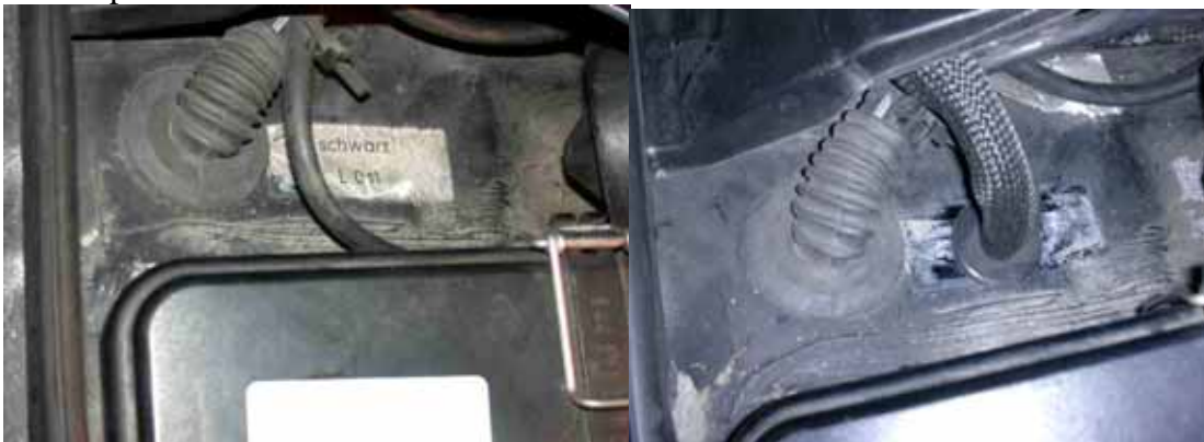
Image 22 - Supplemental positive entry besides fuse/relay box
